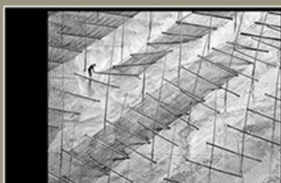
REPAIR NET FRAME 6 H W CHAN, HONG KONG
